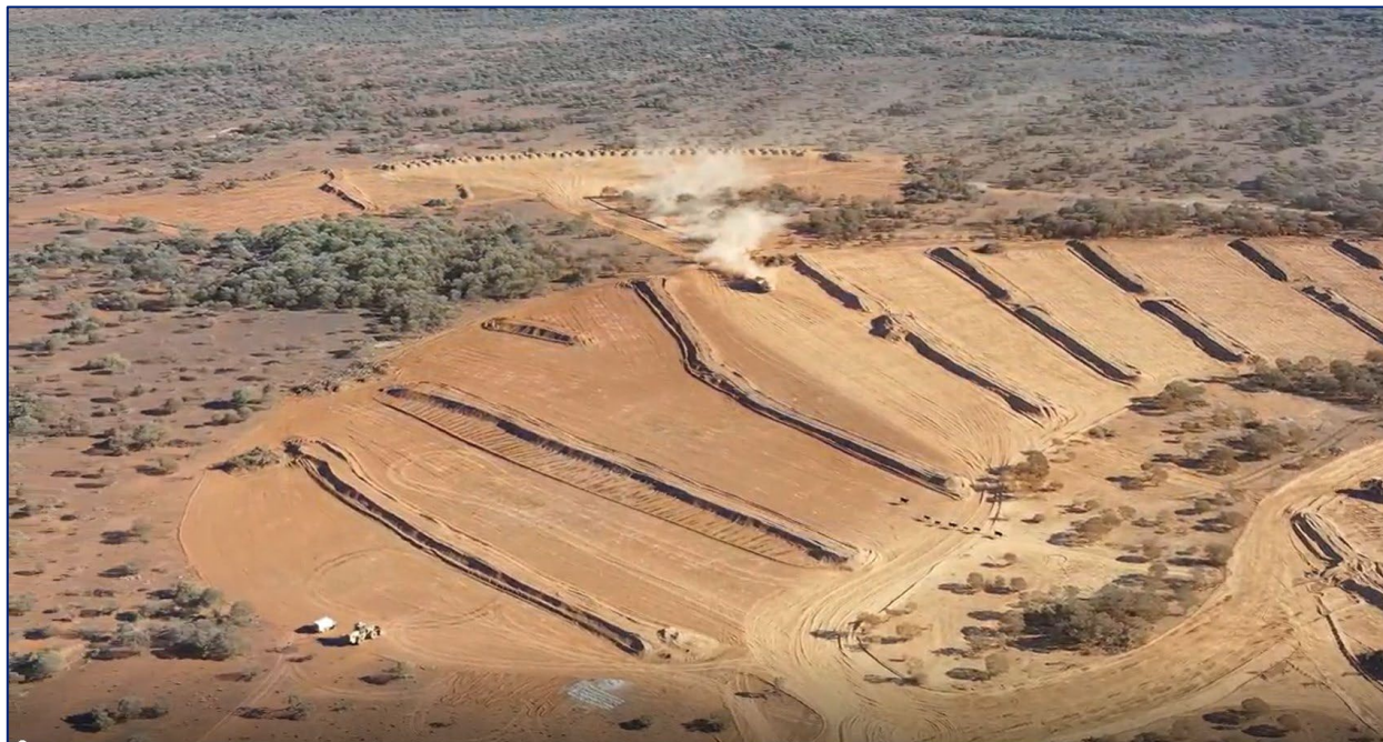
Figure 2: Initial open pit works commencing at Trident; the open pit is intended to take 12 months before commencement of the underground mine
