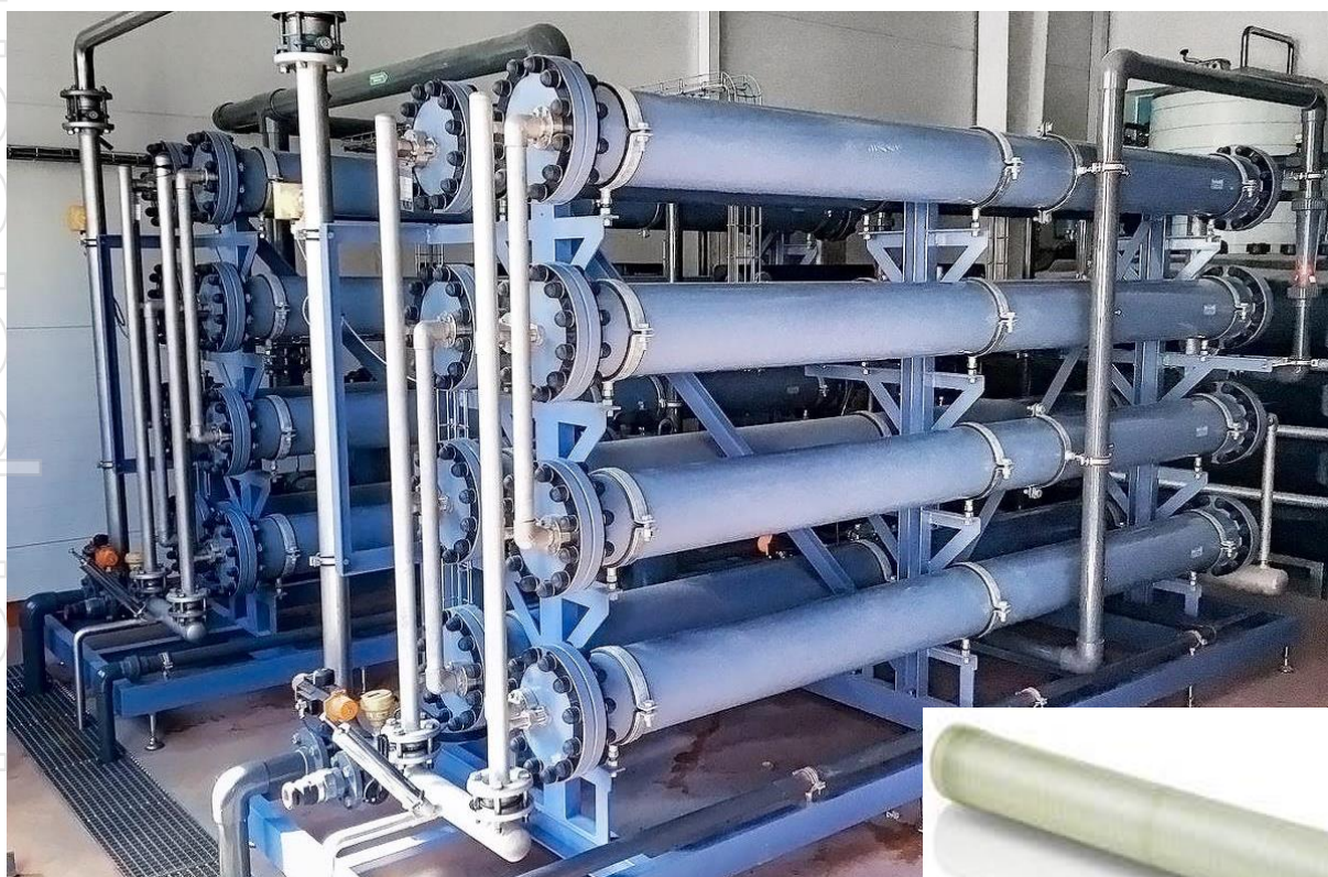
Figure 1: Example of a Nanofiltration system and the membrane utilised
