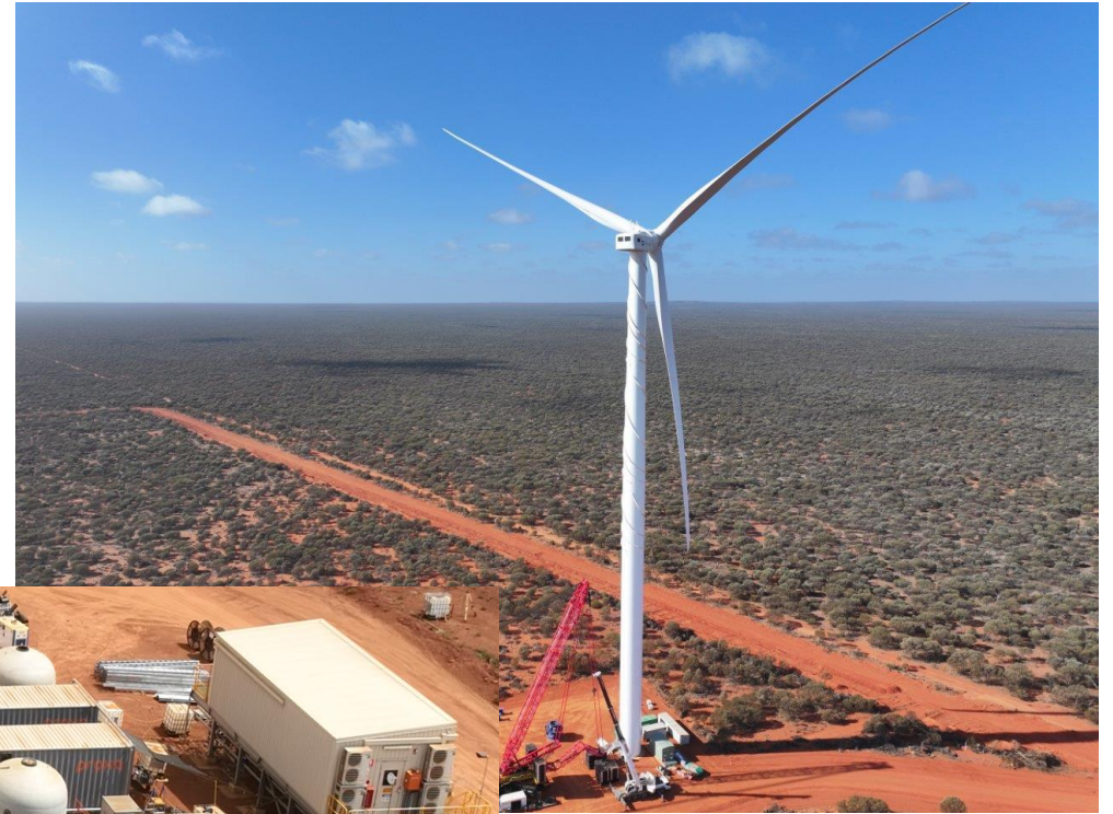
Wind farm - 2 of 4 wind turbines now installed (With our power purchase agreement (PPA) partner, Zenith Energy)
