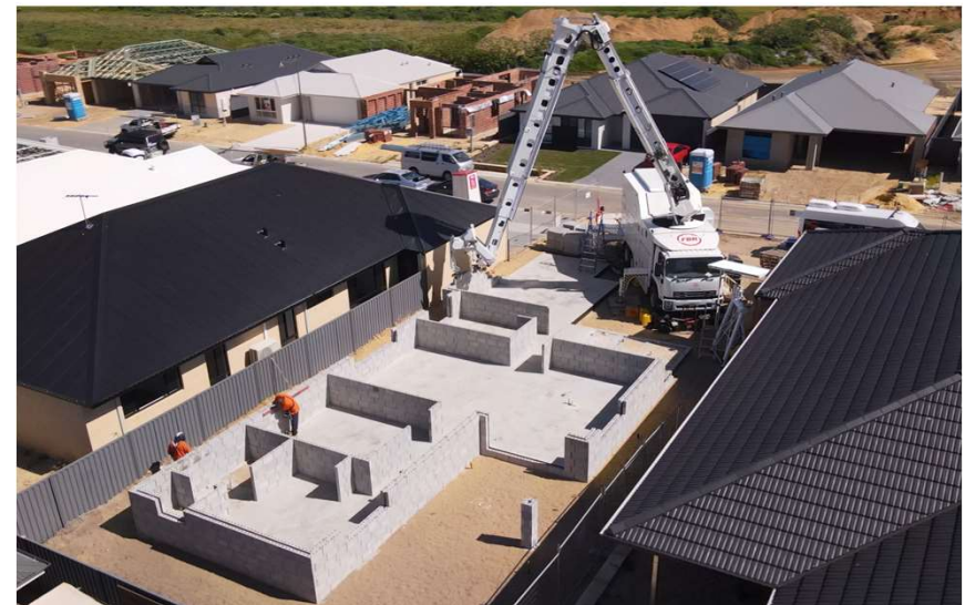
Hadrian X® building a structure in Perth, generating zero on-site masonry waste
