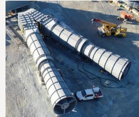
Underground primary ventilation
