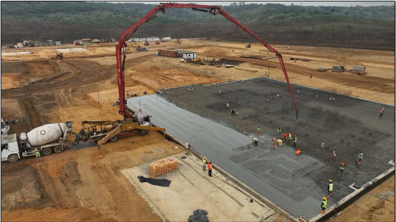
Figure 1 – Subantando Fertilizer Plant, located in Cabinda, Angola – concrete pour for the slab underway.
