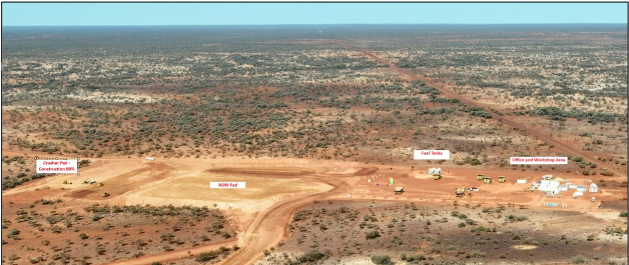
Figure 2 – Aerial view of Crusher Pad Construction, ROM Pad, Office and Workshop Area
