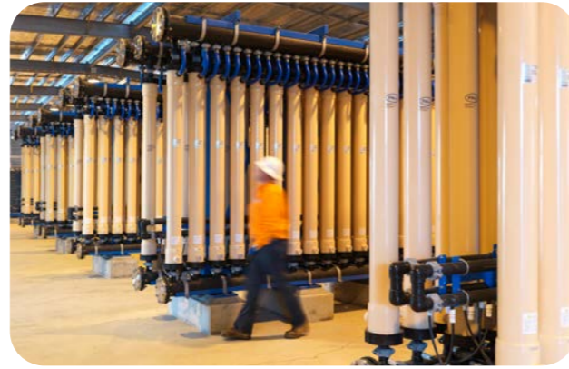
The Talinga Water Treatment Facility uses reverse osmosis to prepare water for beneficial uses such as crop irrigation.
