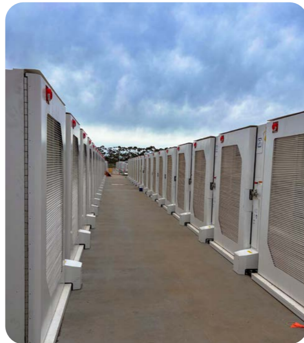
Battery containers at the Mortlake large-scale battery energy storage system.
