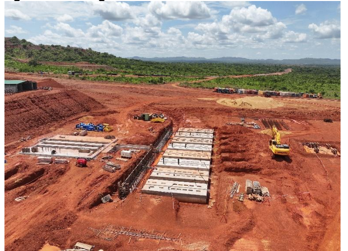
Figure 6: Aerial view of process plant and infrastructure
