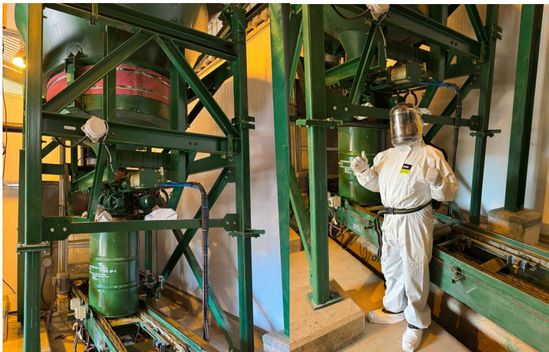
Figure 1 and 2: Yellowcake being drummed at Kayelekera’s packaging and drying plant
