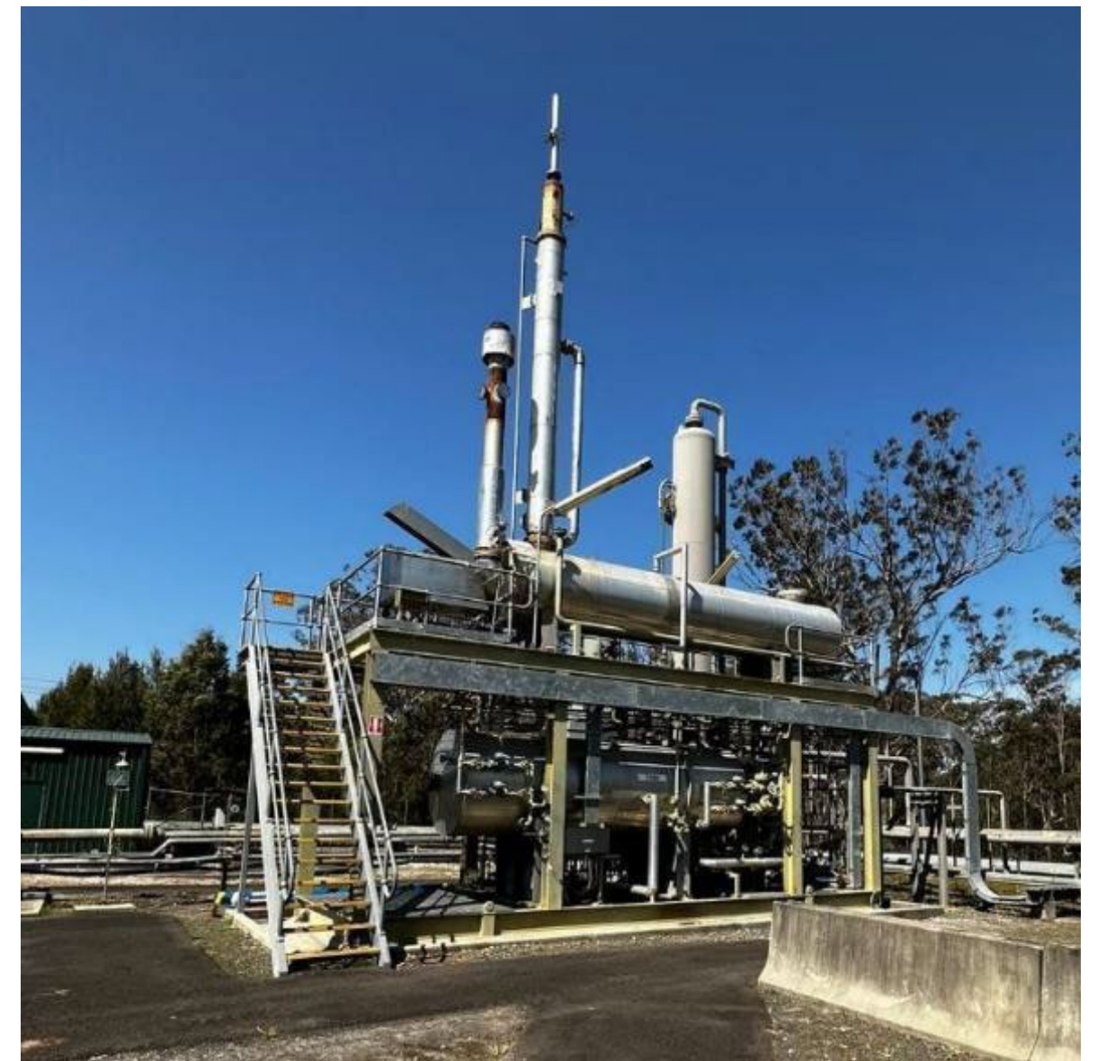
Carpentaria Gas Plant on location in Camden, NSW prior to relocation
