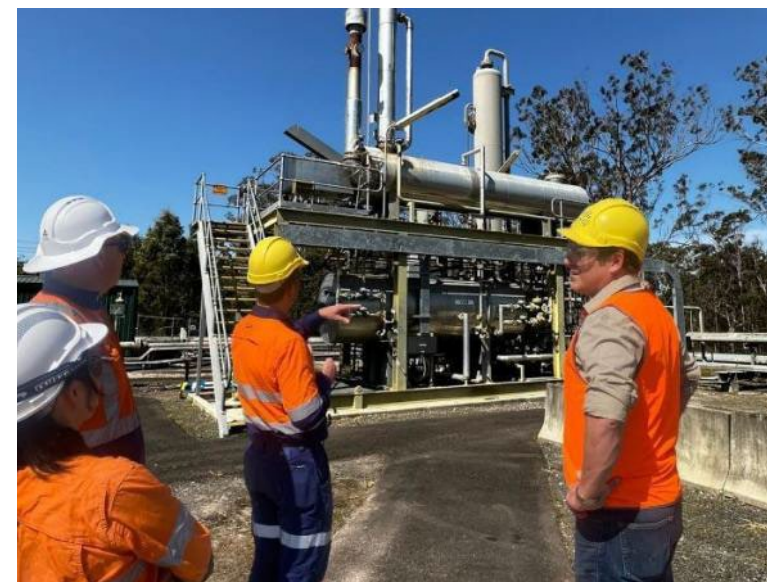
Carpentaria Gas Plant in operation immediately prior to acquisition
