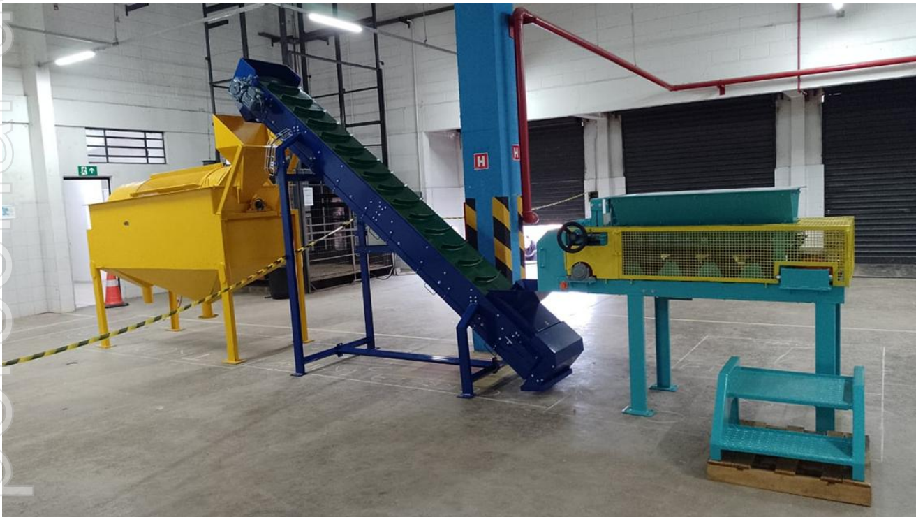
Figure 1: Trommel, conveyor and feeder in order from left to right
