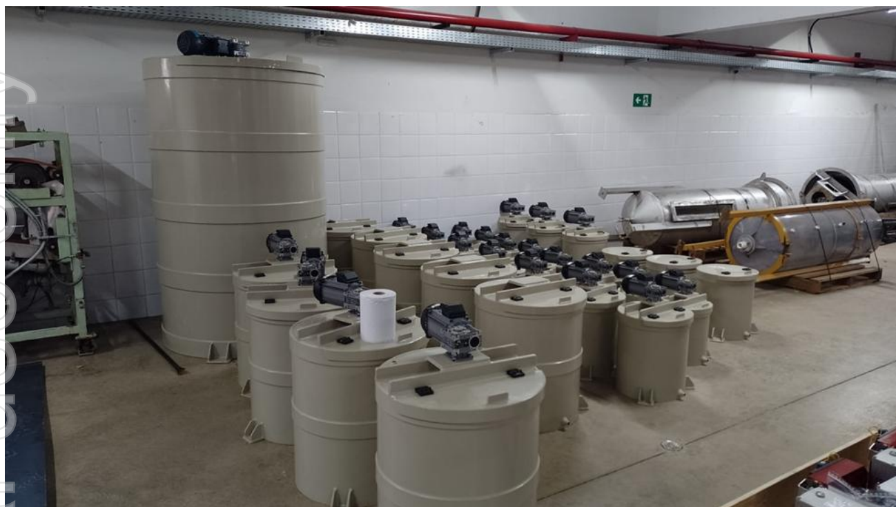
Figure 2: Various holding tanks and Counter Current Decanters (CCDs) and from left to right.
