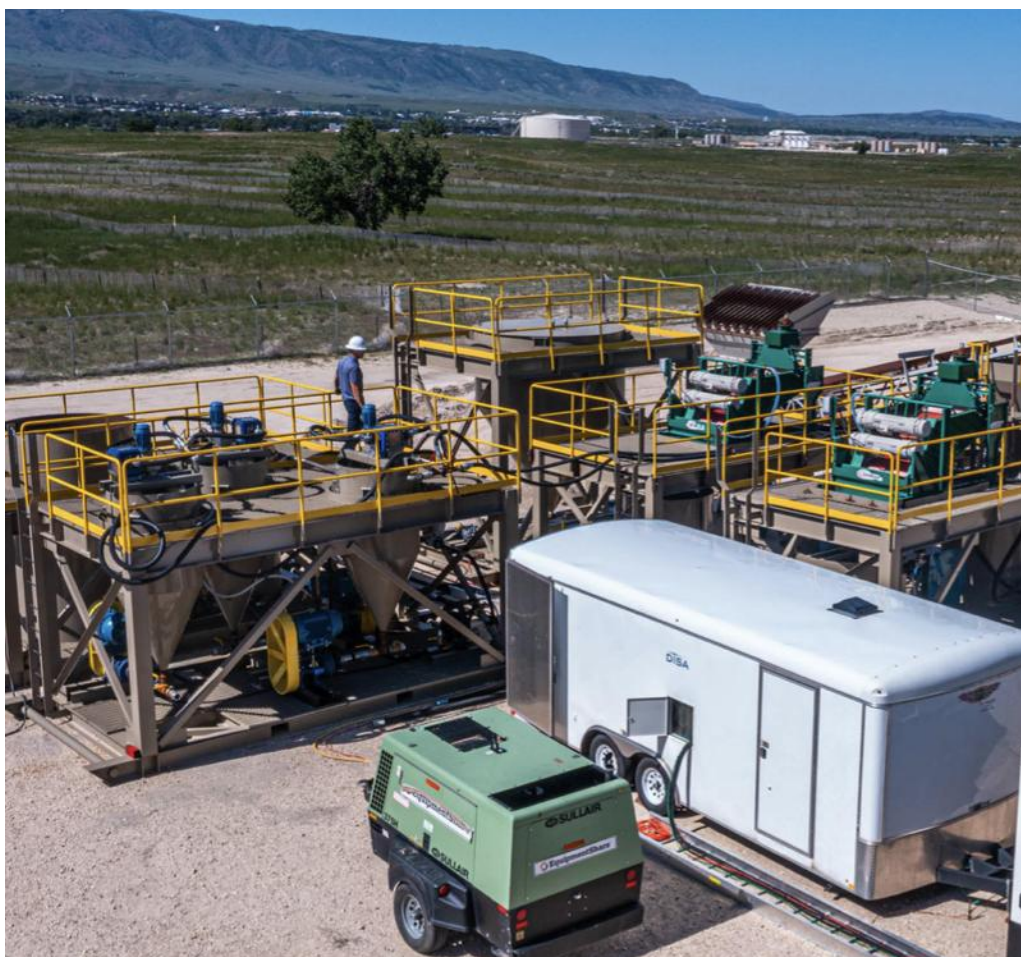
Figure 1 – Example of Gen B modular HPSA components
