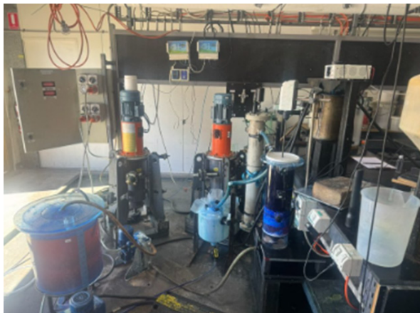
Figure 1 - The BHTC's cobalt solvent extraction circuit.
