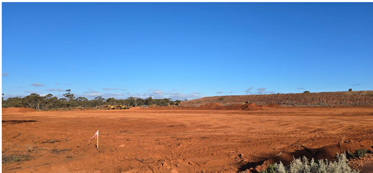
Figure 3: Clearing and topsoil stripping at Fingals workshop/laydown/office area as part of ongoing site establishment activities.
