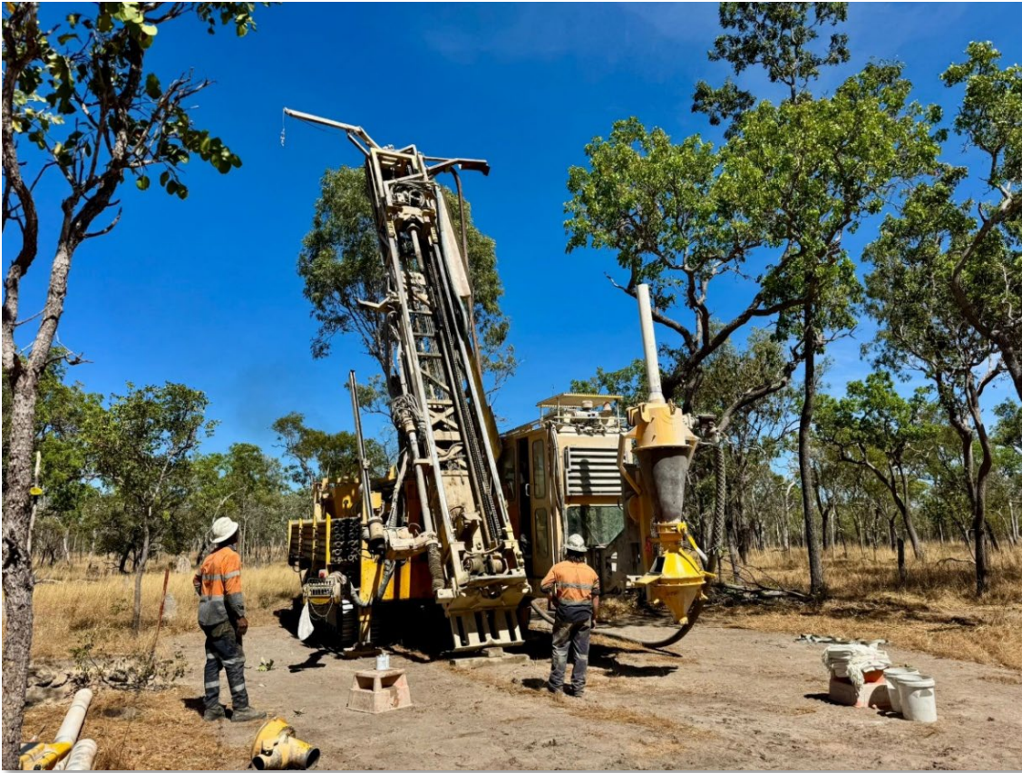
Figure 1: WLRC0001 hole location with RC drill rig being set up over site
