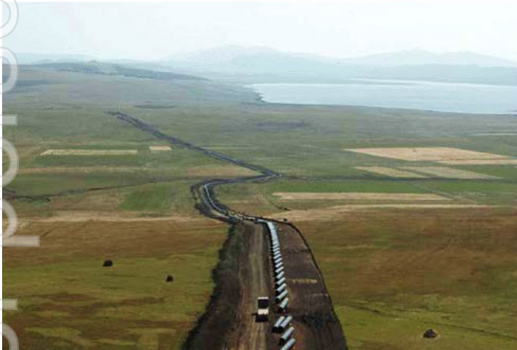
Pipeline construction within terrain similar to that traversed by the CEIP infrastructure corridor on the Eyre Peninsula.
