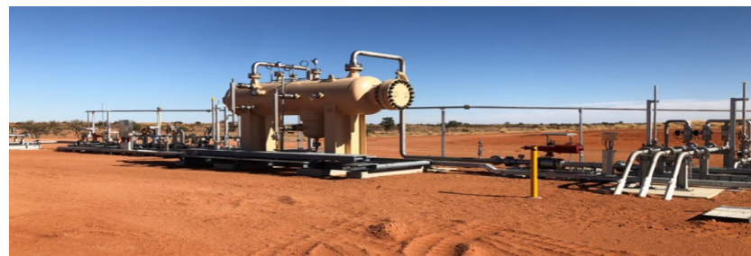
Vali -1 production separator/ infrastructure
