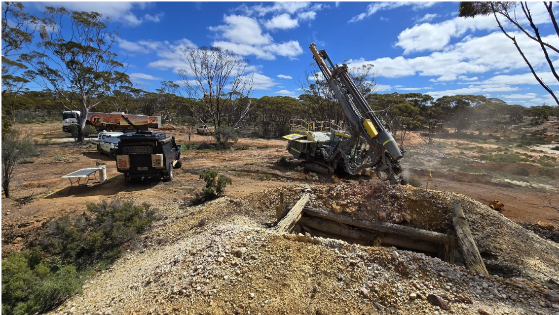
Figure 1: Track mounted RC drilling in progress at the Mt Palmer Gold Project.
