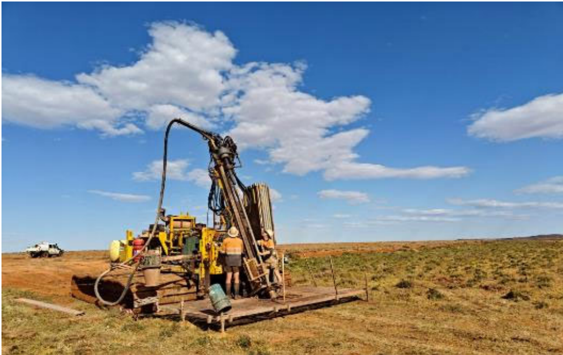
Track mounted lake AC rig, 5km North of Apollo Hill in flat salt lake bed terrain – 10 September 2024.
