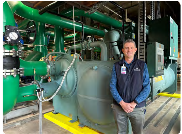
Facility Manager, Ben Watty, alongside Greenslopes Private Hospital's upgraded, energy efficient cooling system.
