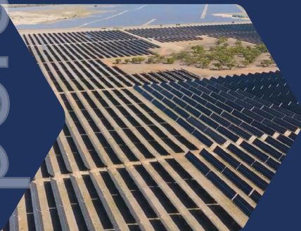
Communications works for Vena Energy at Tailem Bend Solar Farm, southeast of Adelaide, SA.
