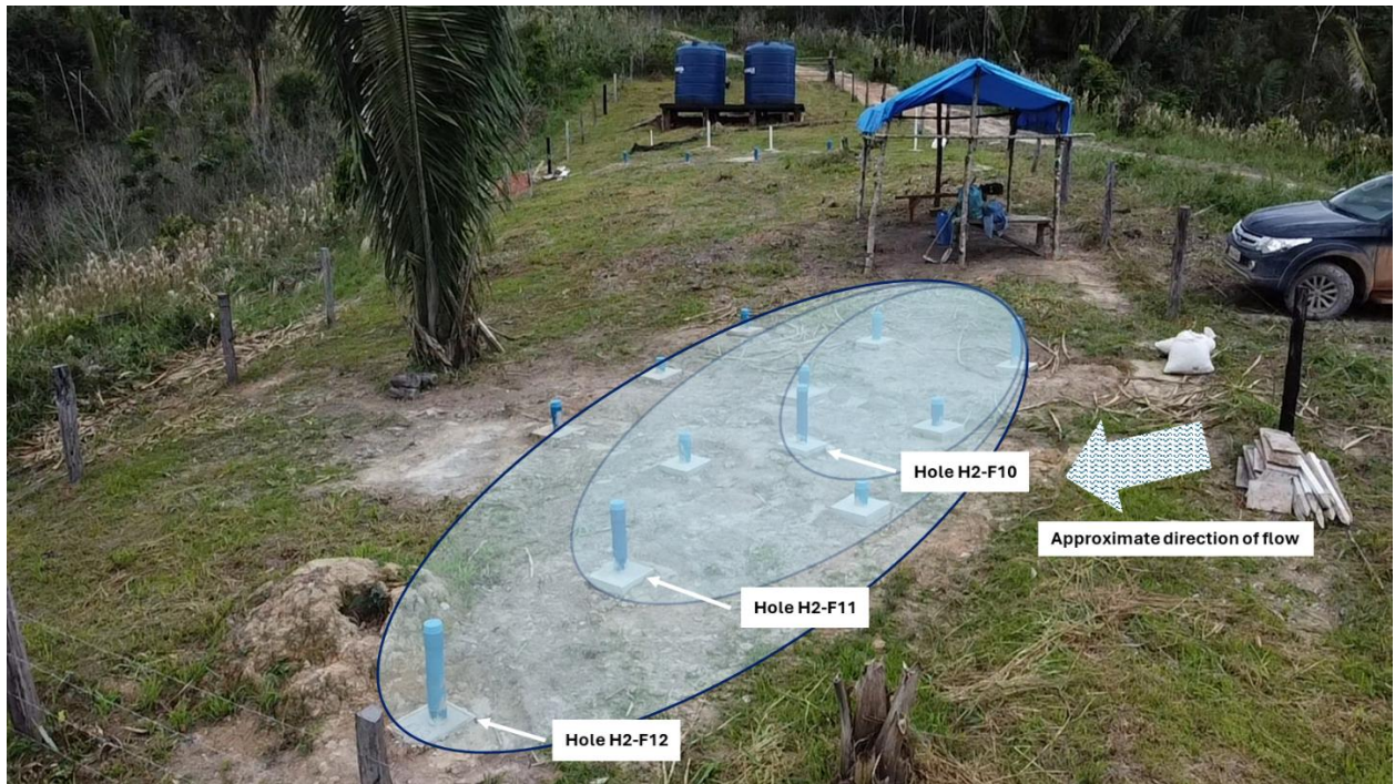
Figure 2. Field pilot trial and setup showing distribution of monitoring holes H2-F10, H2-F11, H2-F12. Rings indicate approximate area of leaching influencing grades received from the PLS, with H2-F10 being the smallest leaching area.
