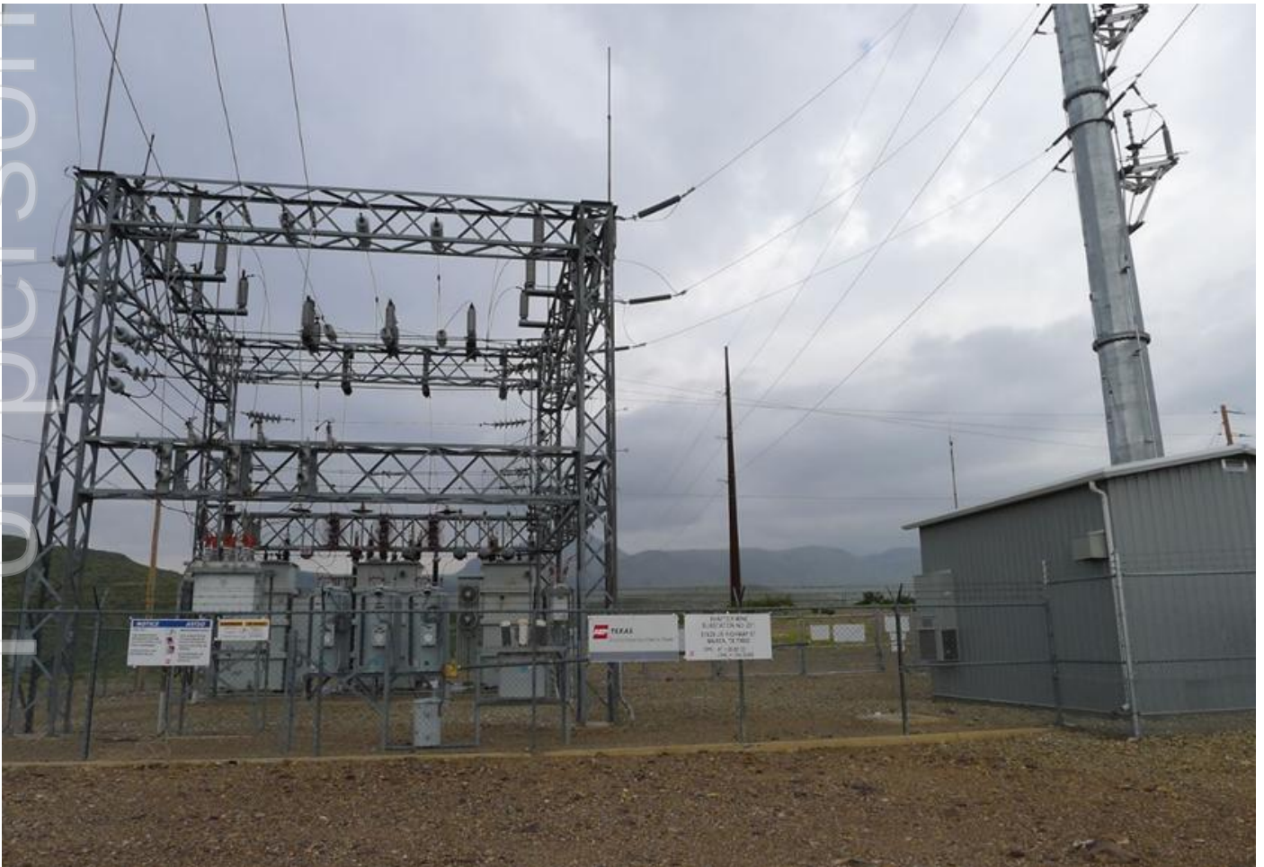
Figure 5: Shafter Mine and Processing Substation.
