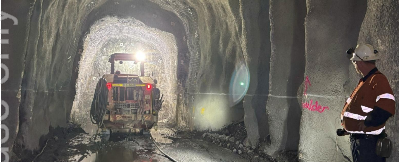
Figure 6. 10100-level access to the high-grade silver Upper North Lode established in September.
