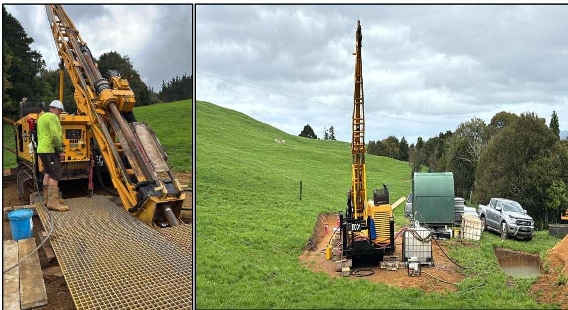
Drilling Hole 1 at Scotia South : Drilling program underway at Waitekauri Gold Project
