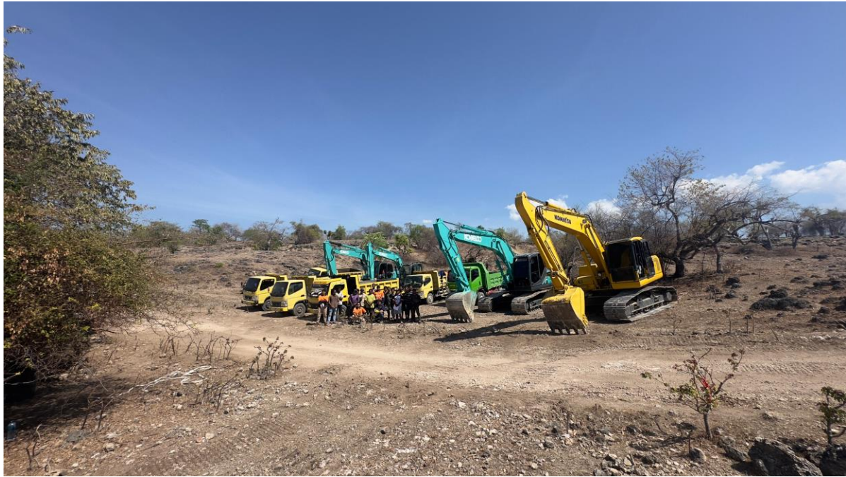
Figure 6: Mobilisation day of contractors to the Werumata Limestone Project to commence drill track and pad preparation.
