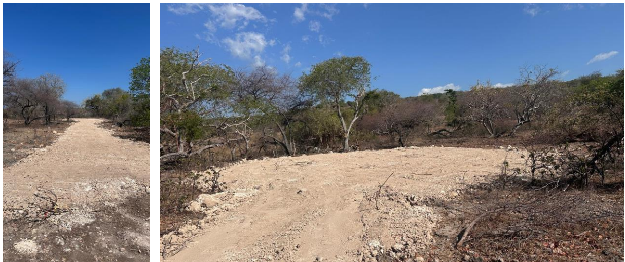
Figure 7: Examples of the work conducted by local contractors at Werumata Limestone Project ahead of drilling
