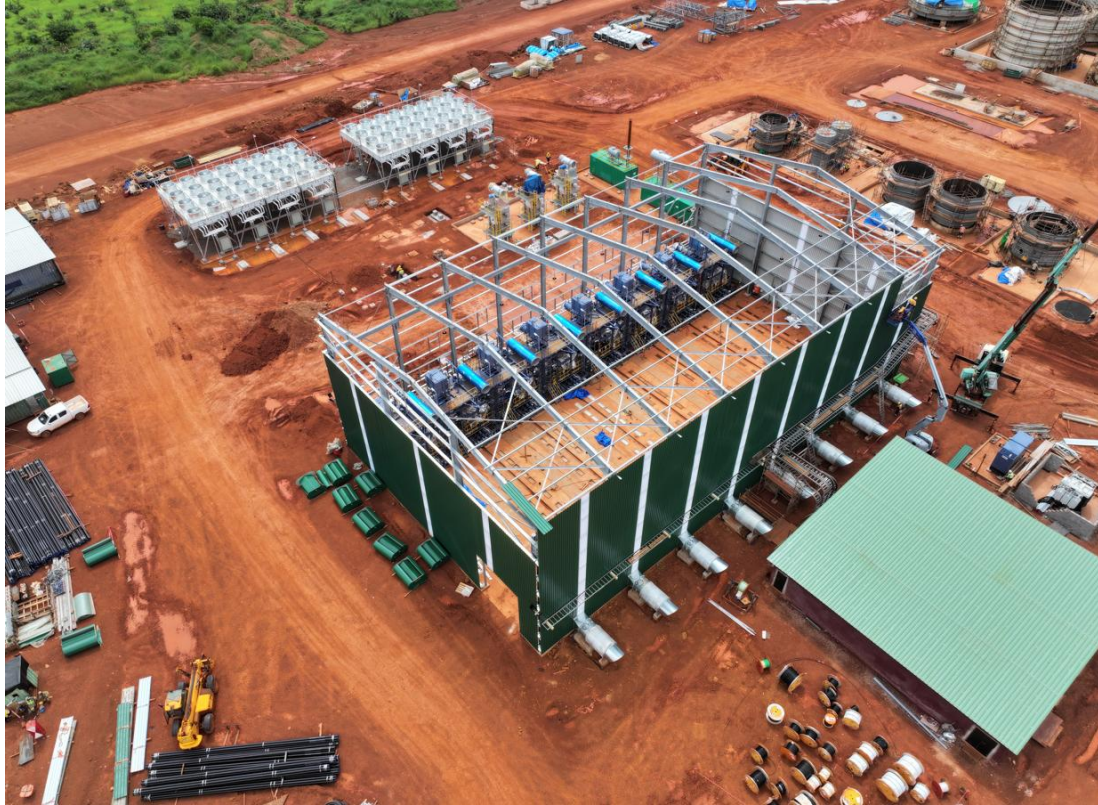
Figure 11: Power station with engine haul building erected and switch room complete (12 October 2025)
