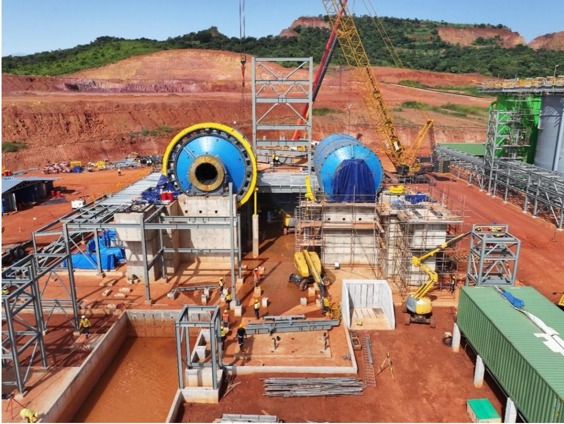
Figure 2: View of milling building showing mill suspended slab complete and mill installation (12 October 2025)
