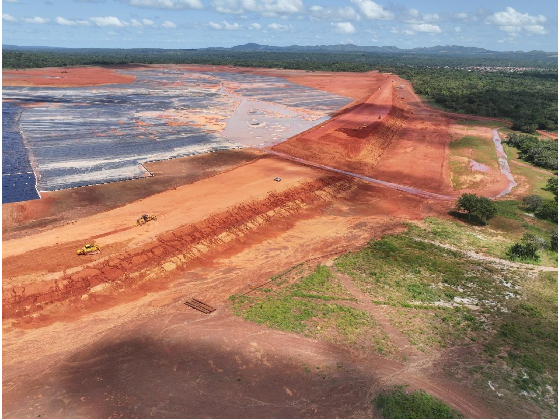
Figure 4: Tailings storage facility showing the extent of lining and main embankment construction (12 October 2025).
