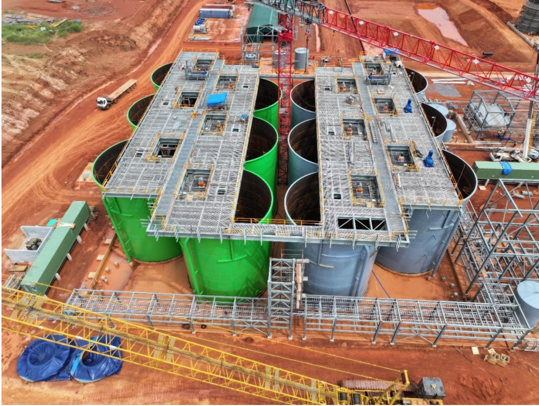
Figure 6: View of CIL with pipe rack and top of CIL tank steel erection (12 October 2025)
