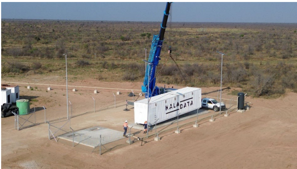
Figure 1: Photo of a Kala Data modular data centre installation, similar to the system proposed for Arrowsmith planned for Q1 2026.
