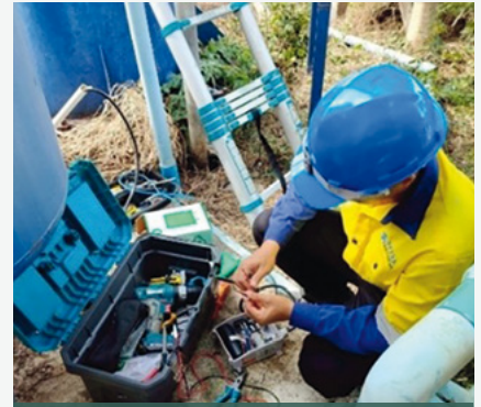
Maintaining 16 water filtration stations
