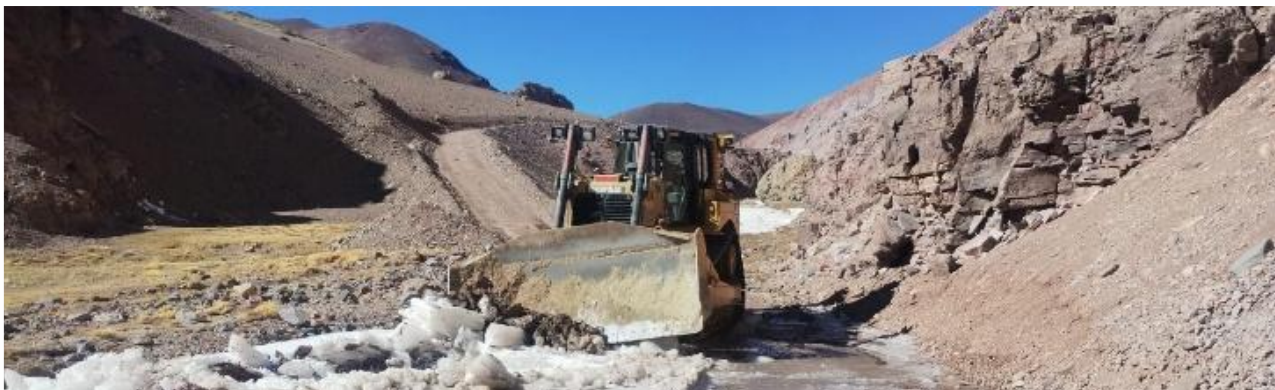
Figure 1 – Bulldozer clearing existing tracks of snow and rock debris en route to the TMT camp.
