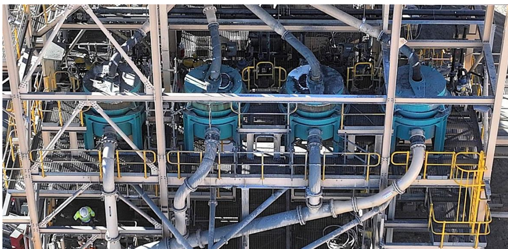
Figure 5: Gravity circuit with full complement of four Knelson concentrators in operation.
