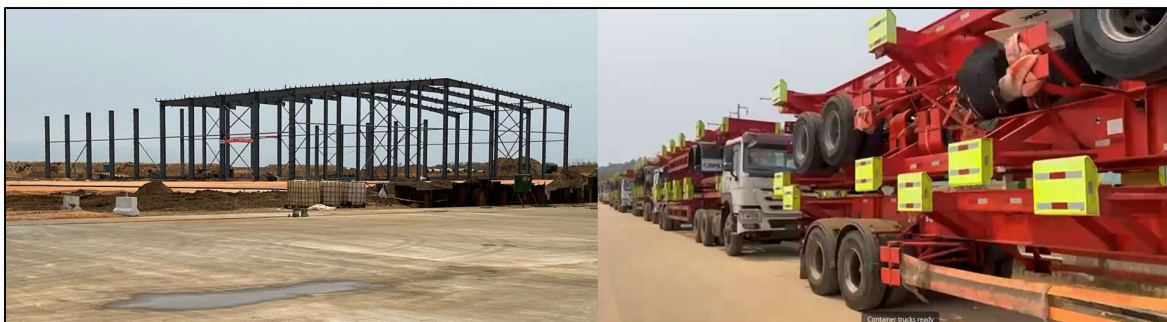
Figure 5: Quay infrastructure under construction and port equipment arriving at Porto do Caio.
