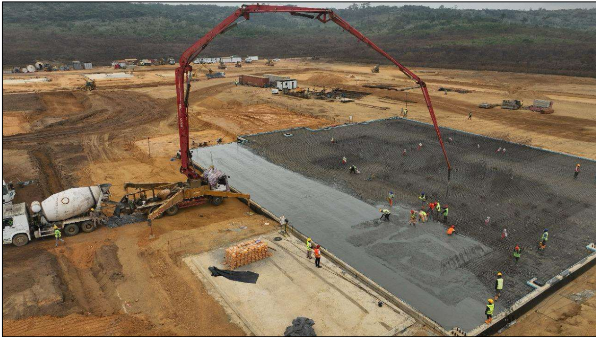
Figure 2– Subantando Fertilizer Plant, located in Cabinda, Angola – concrete pour for the slab underway.
