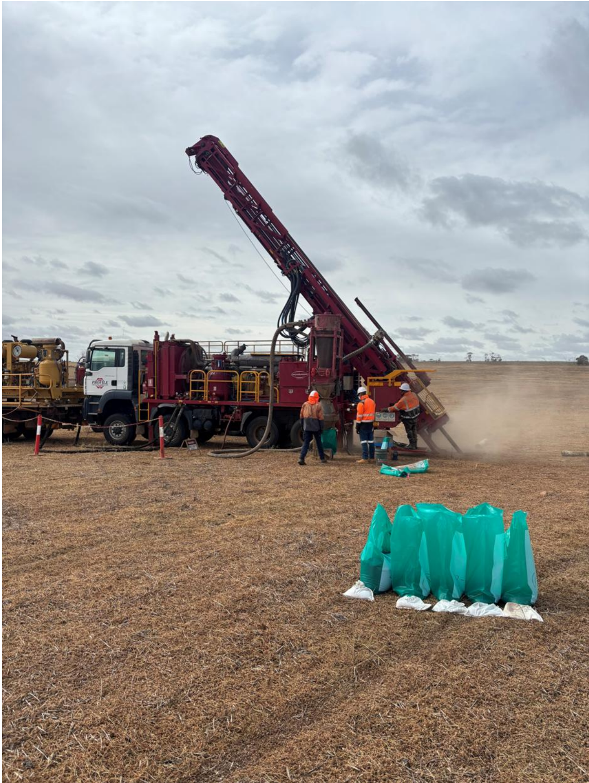
Figure 1 – RC rig on the first hole of the campaign, drilling within the Central Zone.
