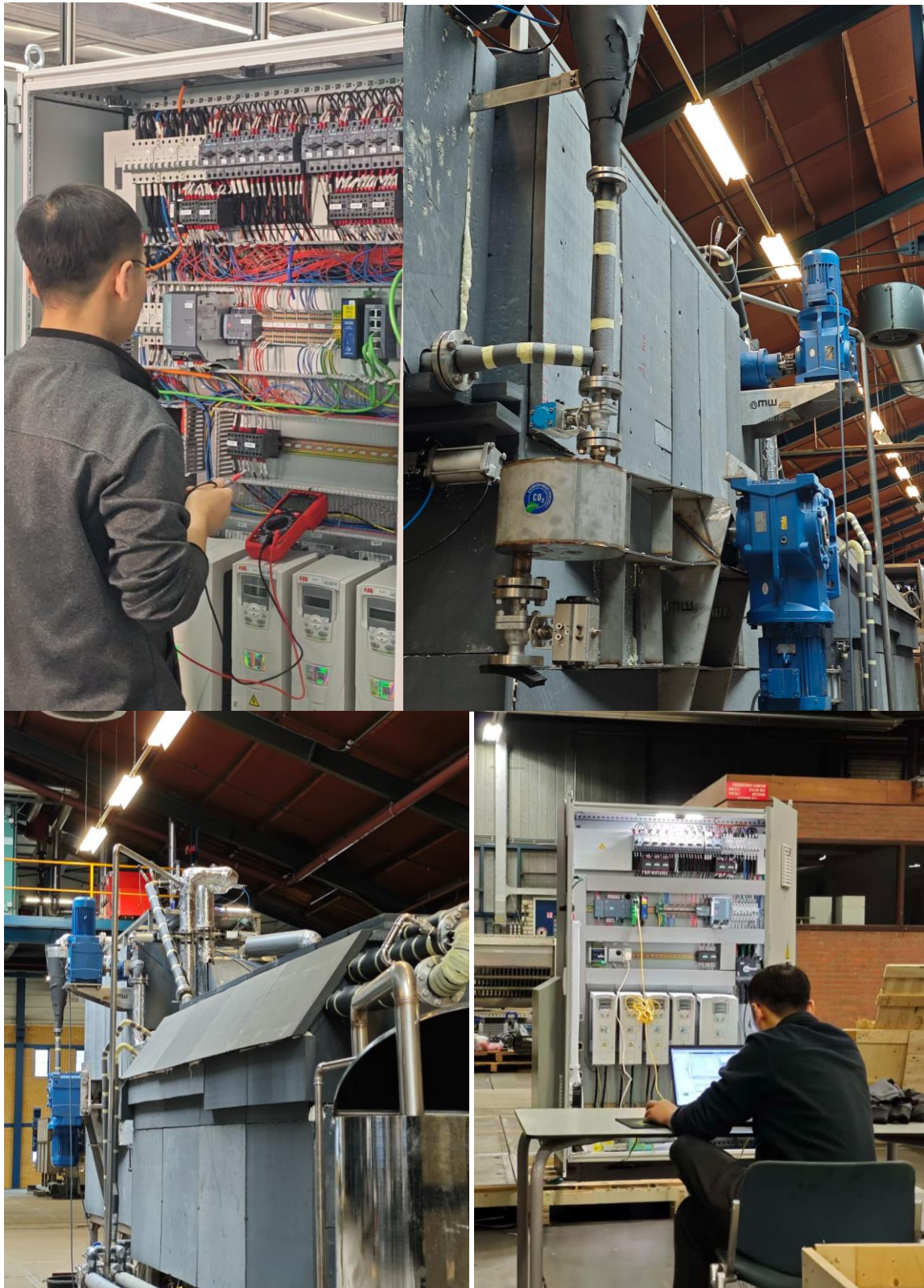
Images: PLC engineer operating the Mest Water control system, full-scale MW installation and control box components; close-up views of the integrated zero-liquid discharge (ZLD) system in operation.
