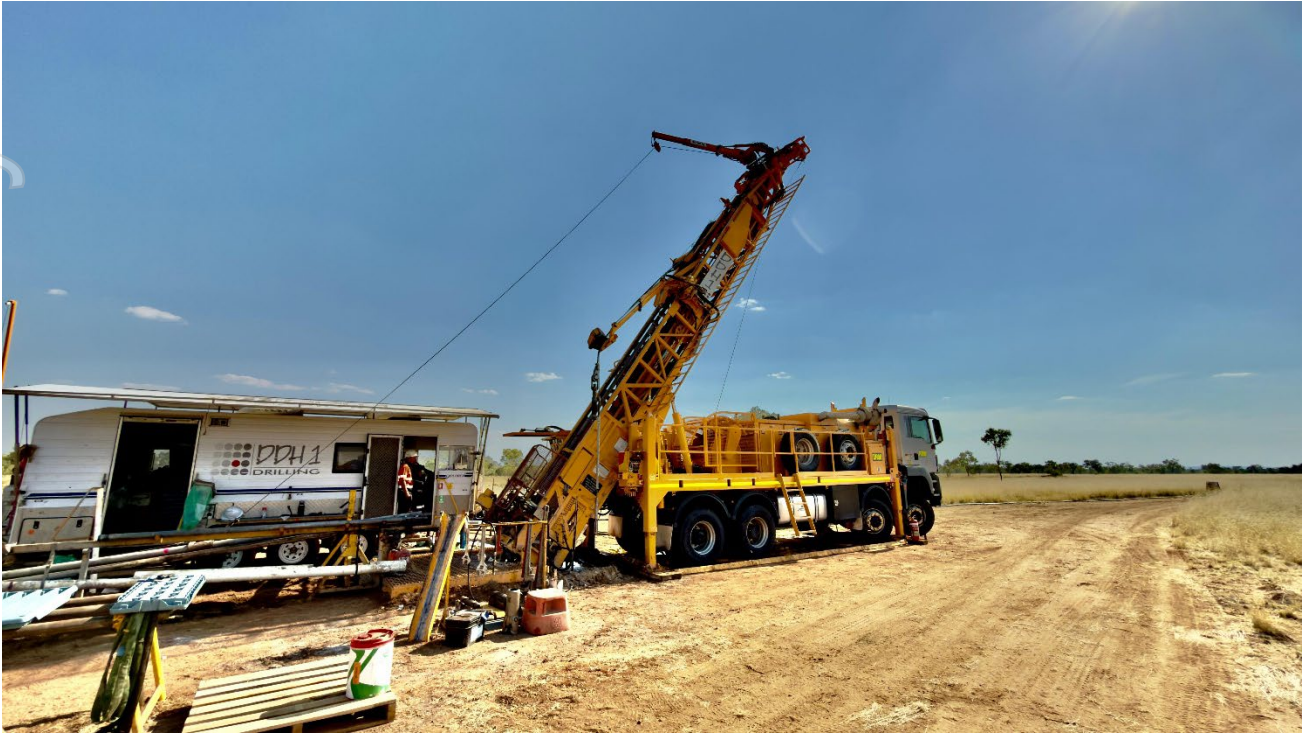
Figure 2. DDH1 drill rig 8 drilling the first hole of the new 2025/2026 campaign at Maronan
