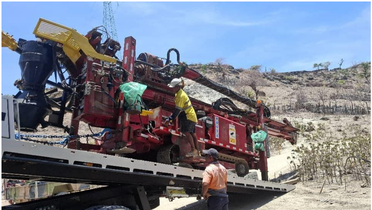
Figure 2. RC drill rig unloading at Werumata staging point in preparation of commencement of drilling
