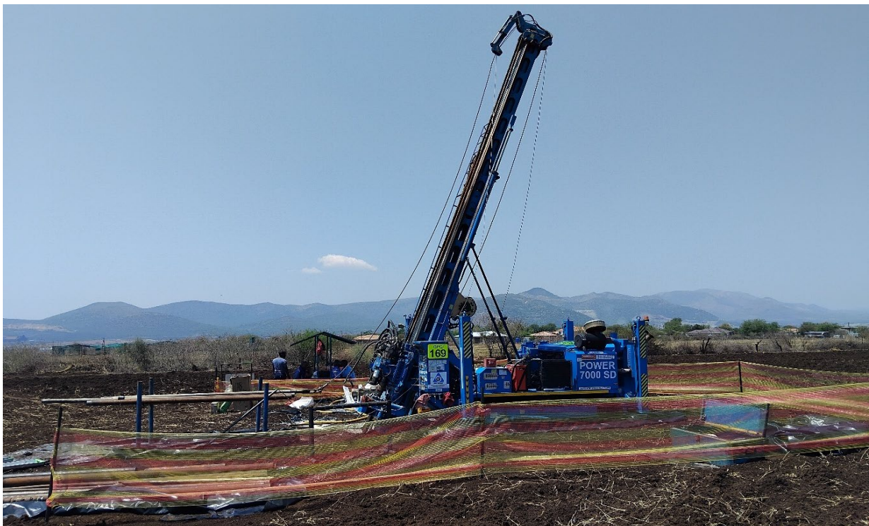
Figure 1: Hanjin P700 Drill Rig in operation as part of DFS drill works program
