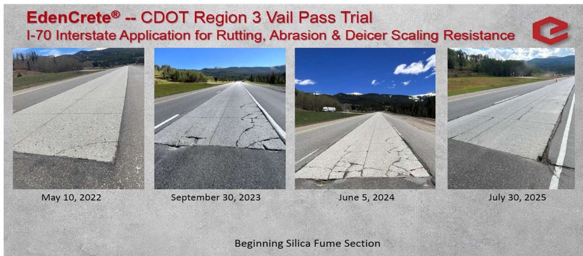
Figure 8. Silica Fume concrete – Beginning Section (in 2025, 2 panels were replaced with bitumen for safety reasons)
