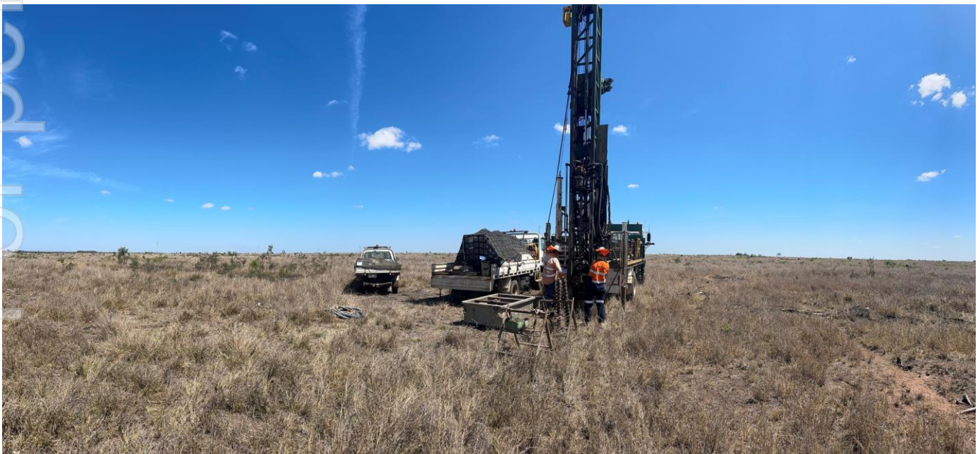
Figure 3: Geotechnical soil sampling along proposed pipeline route to confirm soil and rock technical parameters for design and construction work
