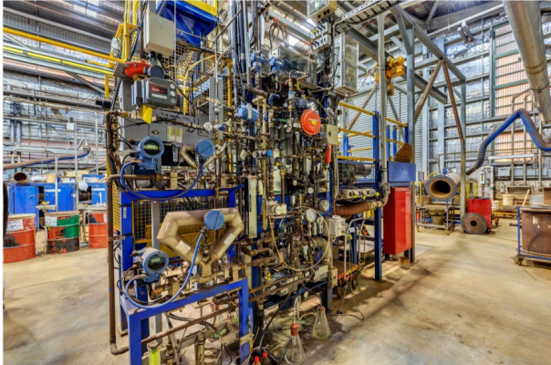
Figure 2: CSIRO Sintering & Pelletising Facility
