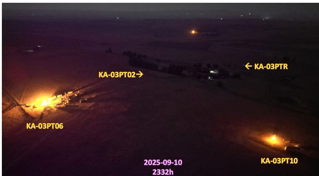
Figure 3: Production Test Well KA-03PT06 being choke tested with ongoing flow testing at well KA-03PT10 (the two other wells are shut in)
