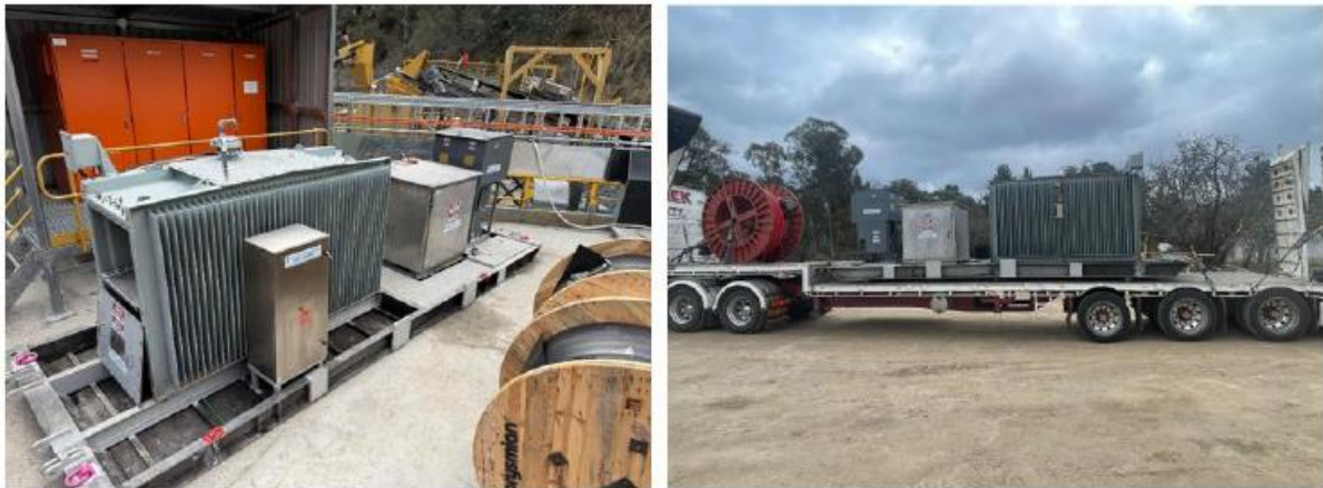
Image 2: High voltage (11 kV) transformer installed next to power station at the Reward Gold plant
