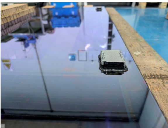
New internal thermal bridge junction box installed prior to double glazing and testing.
