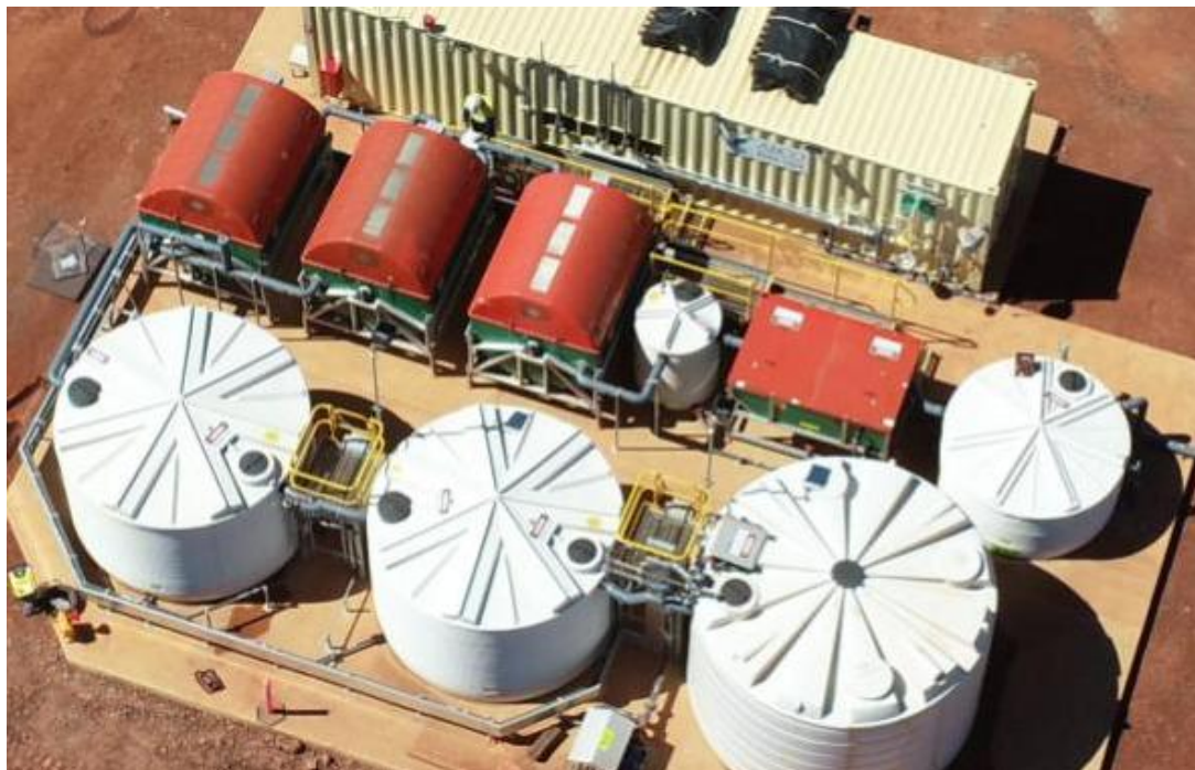
Figure 21: Example RBC type WWTP installed at Newmont Tanami Operations, NT (Ref: ABCO)
