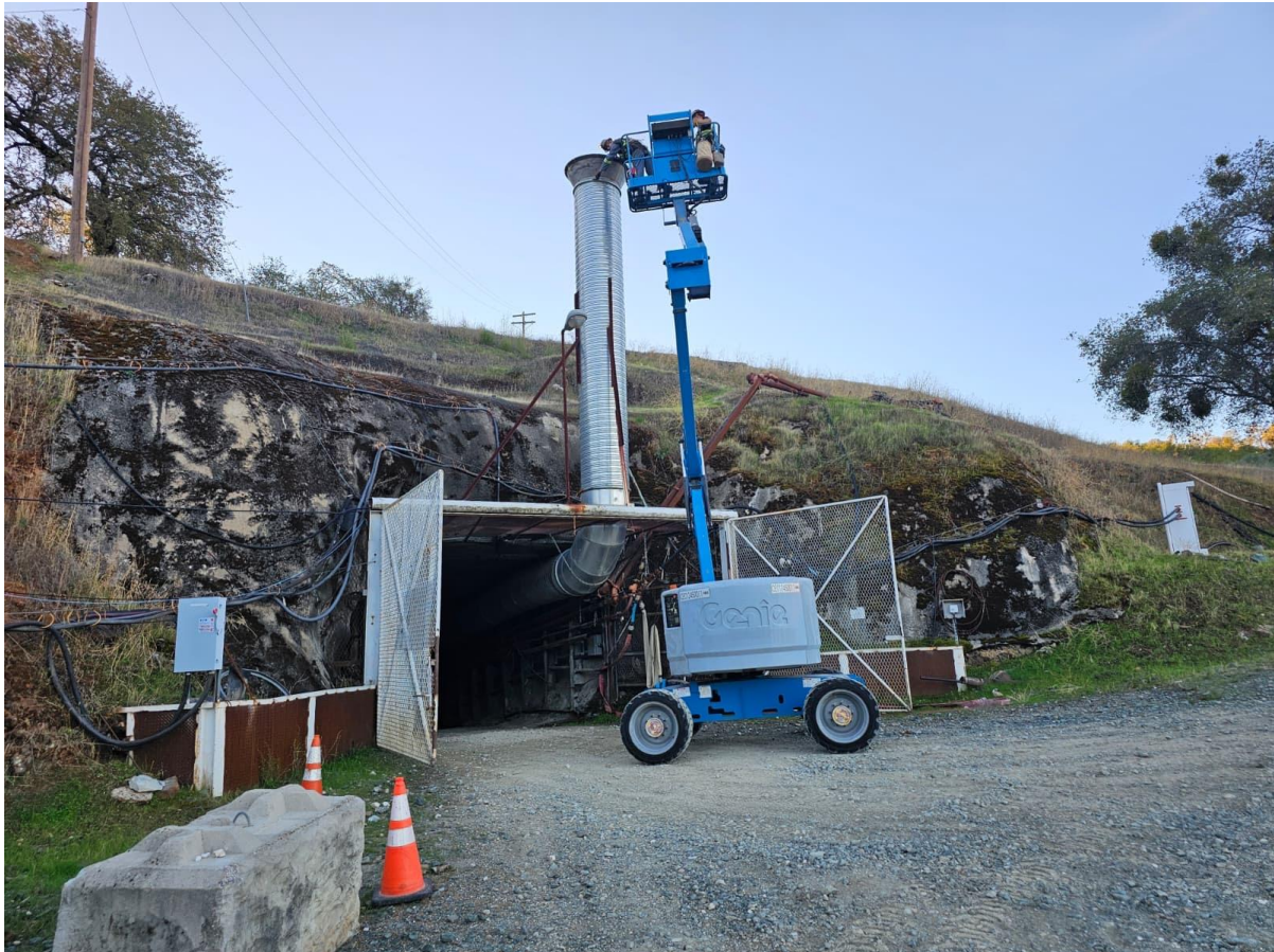
Figure 4: Recently purchased 4x4 articulated boom checking ventilation tower at Stringbean Alley Decline portal.
