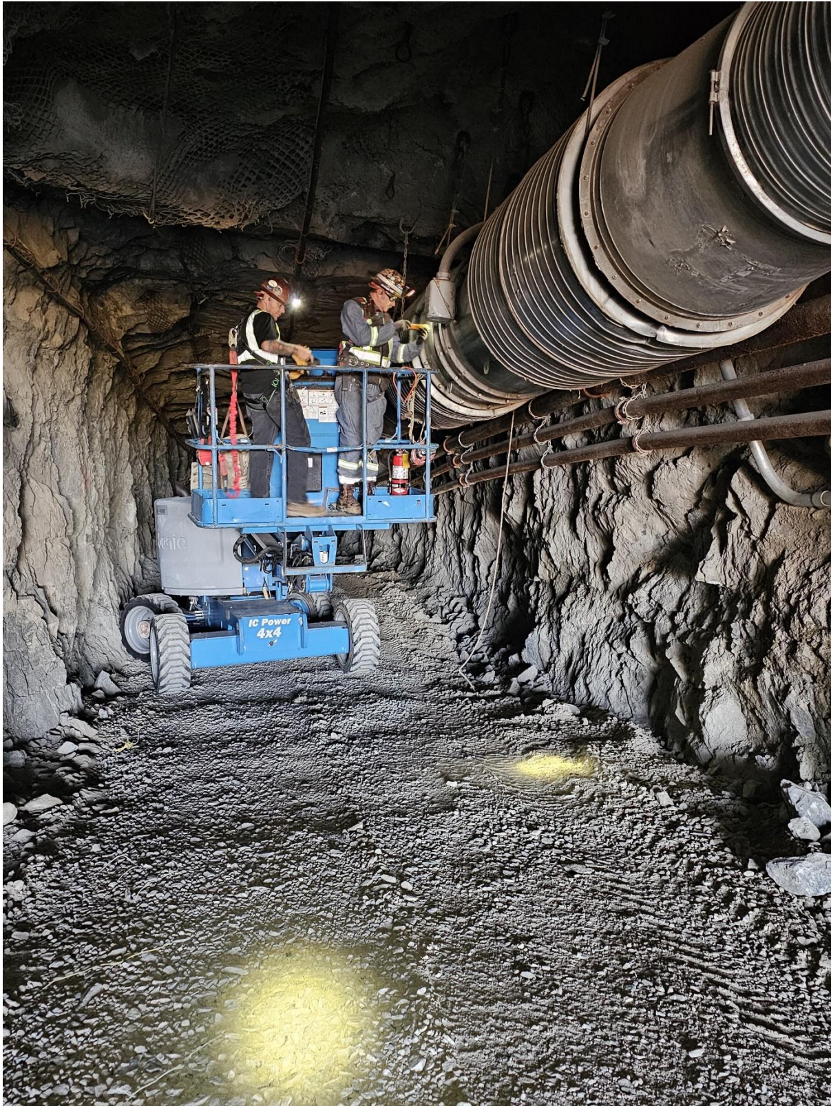
Figure 5: Recently purchased 4x4 articulated boom performing checks on ventilation fan at Stringbean Alley Decline portal. The work platform provides a stable platform as the Company advances pumping equipment and drops ventilation at the water interface.
