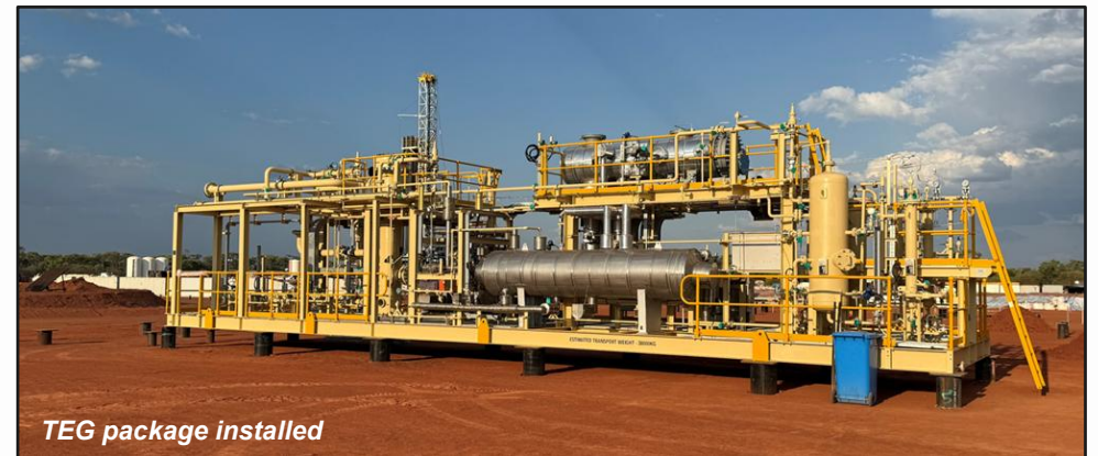
Compressor units installed on SS2 pad
