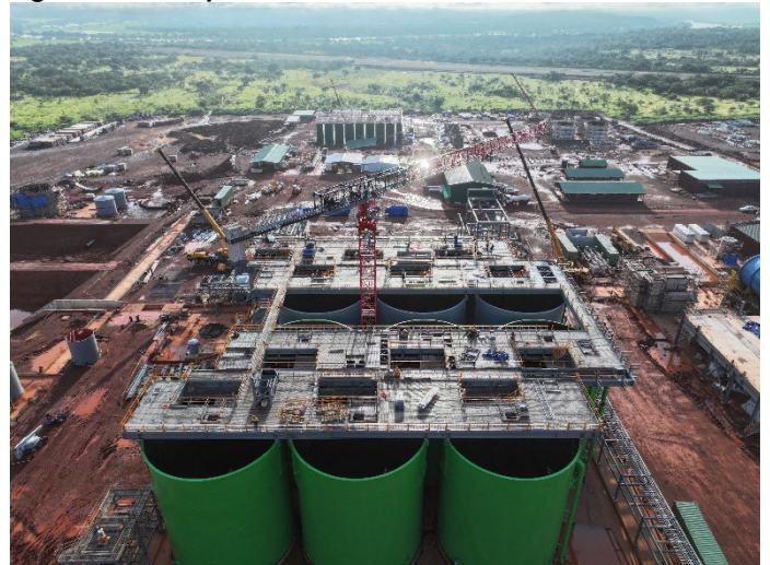
Figure 4: CIL Tank Train A & B
