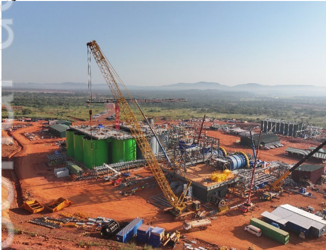
Figure 3: Milling & CIL Tank Train
