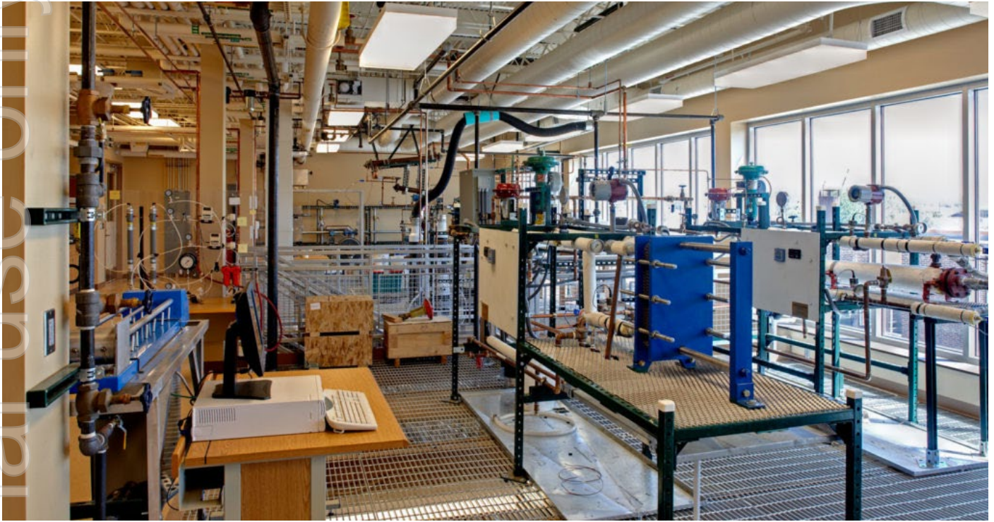
Figure 1 - South Dakota School of Mines & Technology - Chemical & Biological Engineering / Chemistry (CBEC) facilities.
