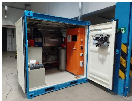
Figure 9 – Filtration unit installed
